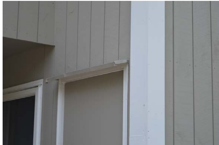
Figure 33. Rain Shield over exterior closet
