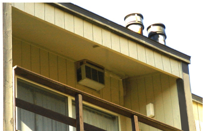
Figure 1 AC unit over sliding door
