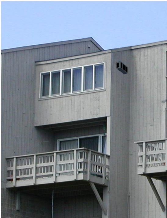
Figure 2: AC unit location at sidewall of Type 'B' unit.
