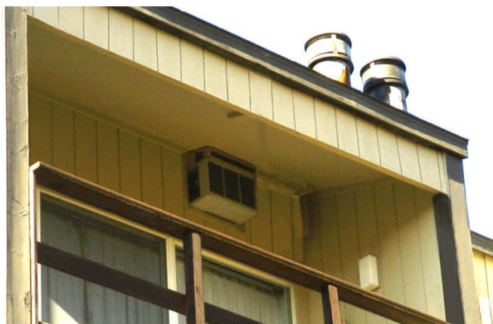
Figure 1 AC unit over sliding door
