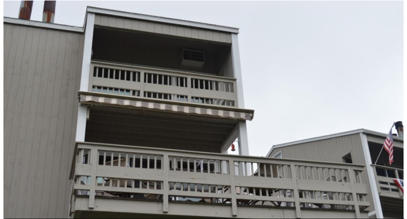
Figure 11. Original top, bottom and intermediate rails with balusters applied to inside face
