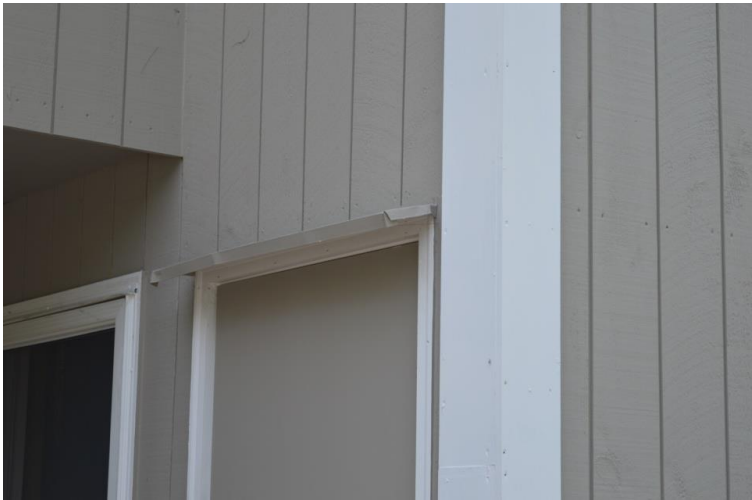
Figure 31. Rain Shield over exterior closet
